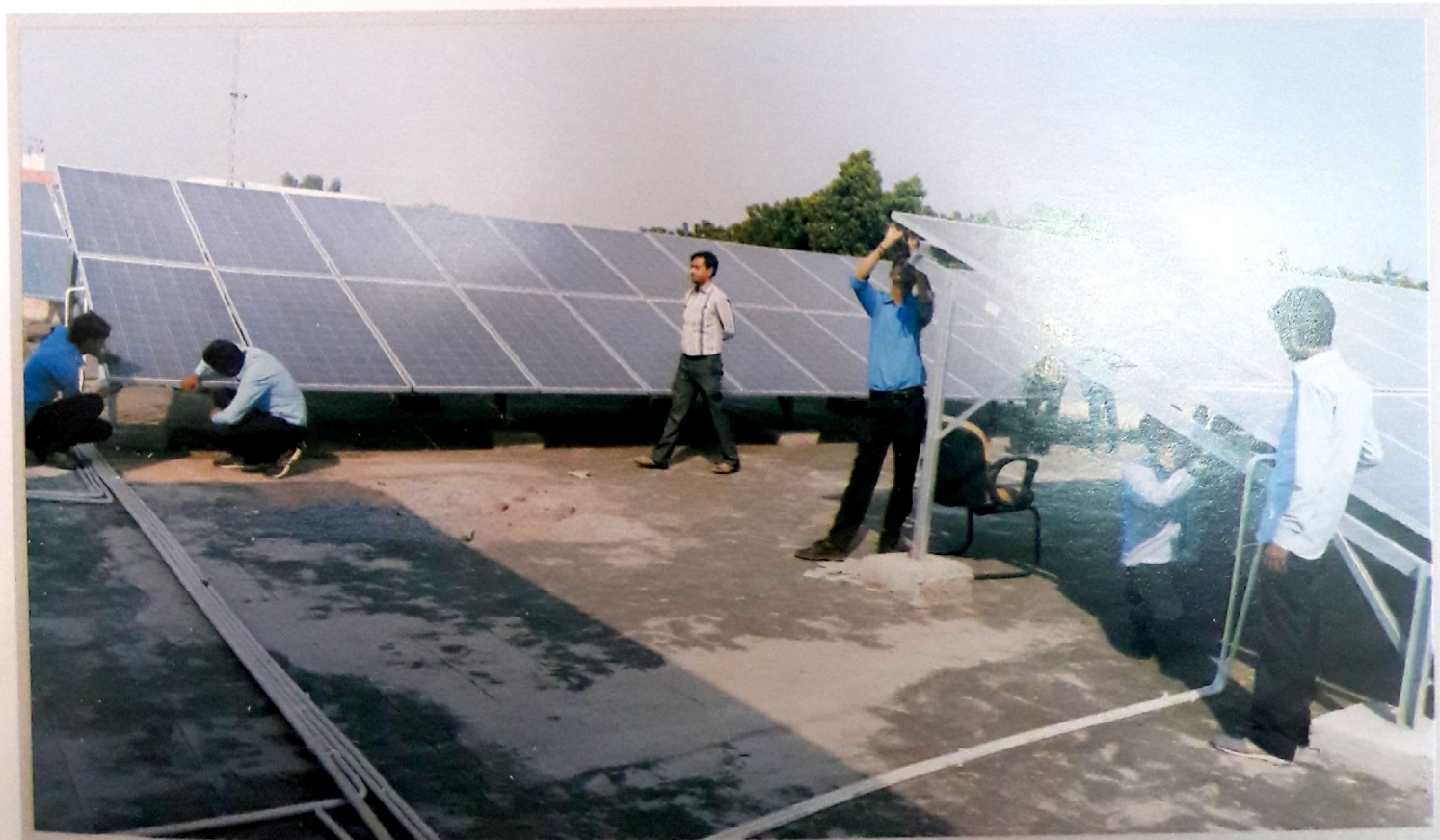
ROOF TOP SOLAR SYSTEM
